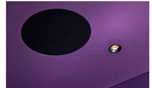
Surround speakers are built into the bespoke ceiling coffer
