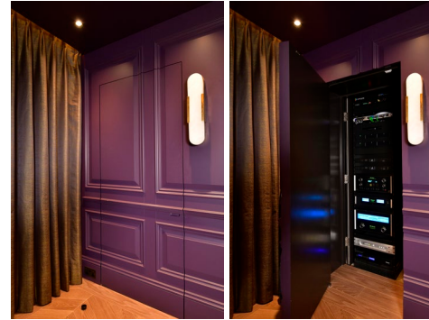
The cinema equipment rack resides behind a 'secret door' in an air conditioned plant room
