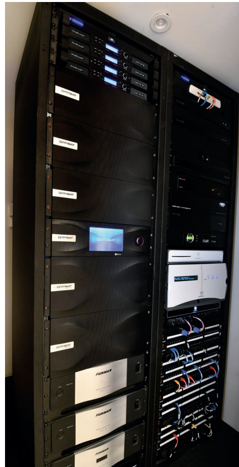
AV equipment racks were completely rebuilt to meet Cyberhomes exacting standards; ensuring reliability and easy servicing and upgrading
