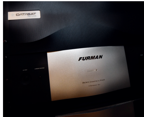
Extensive power conditioning ensures optimum equipment performance
