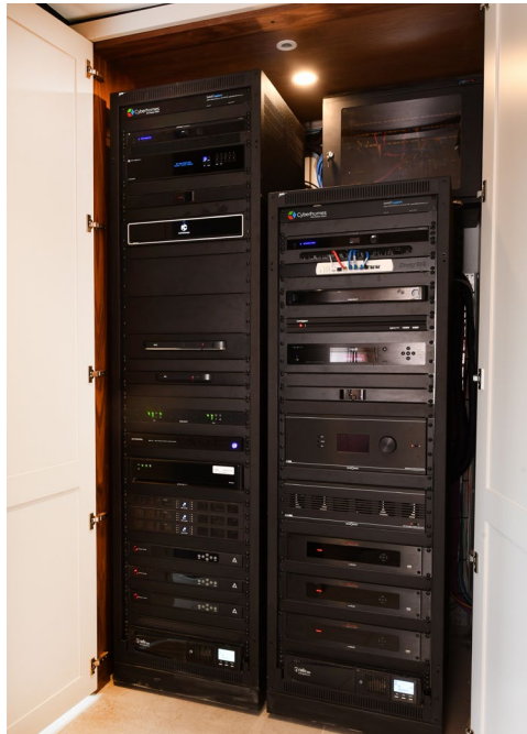
Dedicated AV racks keep equipment out of the living spaces.
