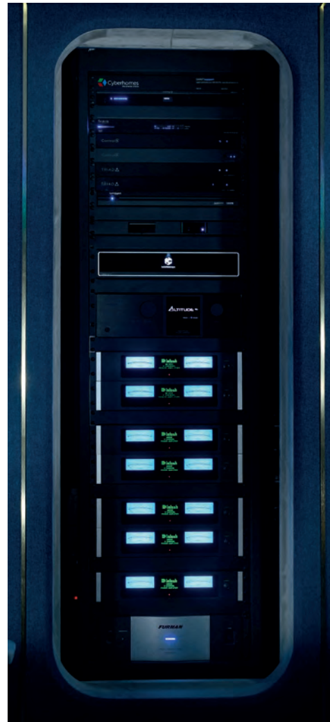
The AV rack is showcased as a feature of the SMARTcinema demo room. We also created easy access behind the rack so visitors can examine the impressive rack building and cabling skills of our engineering team.
